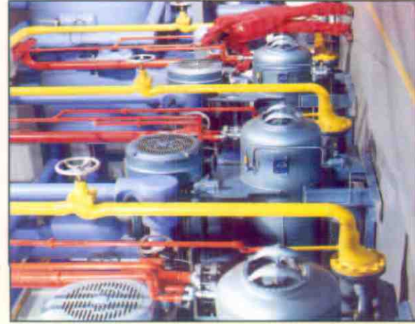
Pumping installations, pipelines and purification plants are all engineering installations.
